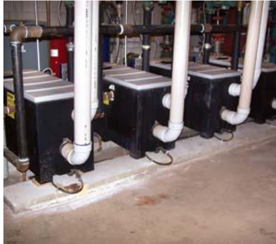
These boiler units at Pellston Middle School/High School were installed as part of an energy-saving mechanical upgrade project in the district three years ago, replacing a single larger boiler. Depending on the demand for heat and hot water, the compact gas-powered units can run individually or in conjunction with one another — allowing for better efficiency. (Ryan Bentley/News-Review)
